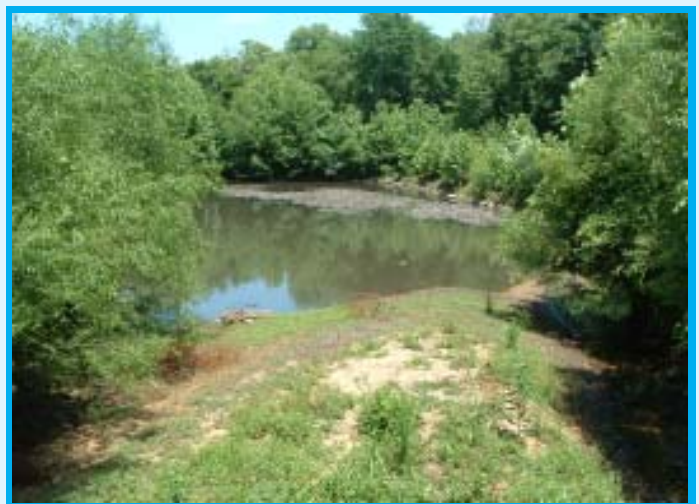
SEDIMENT EVIDENT IN FOREBAY (2008)
